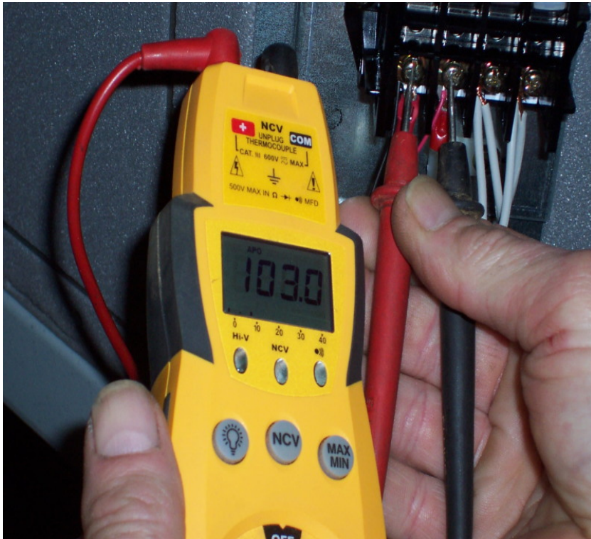
Indoor unit at U1 & U2 communication line
